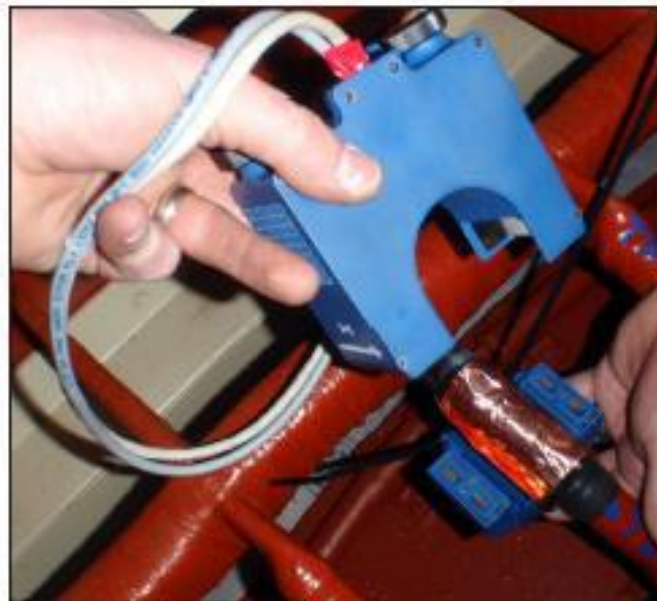
Figure 7: Assembling a Current Transducer Head on a winding link of an Electrical Generator Stator. Reprinted by permission from the USBR.
